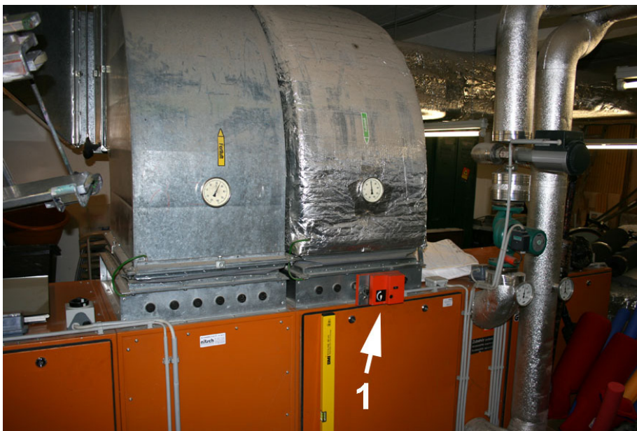
Figure 46: Ventilation system with part for supply and exhaust air. (1) Display for air circulation (see next image)
