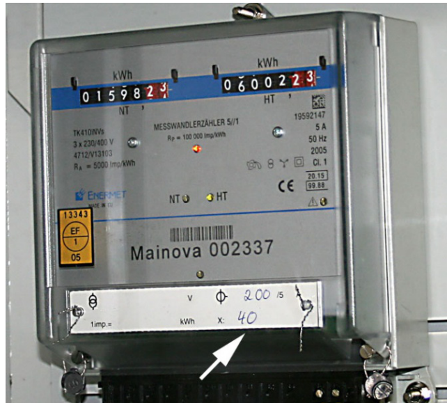
Digital electricity meter with converter for high connected loads (factor = 40 – arrow)
