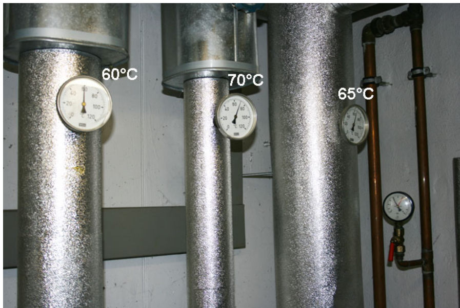
Figure 42: Distribution in the heating circuit in the boiler room with low differences in temperature between the flow and return
